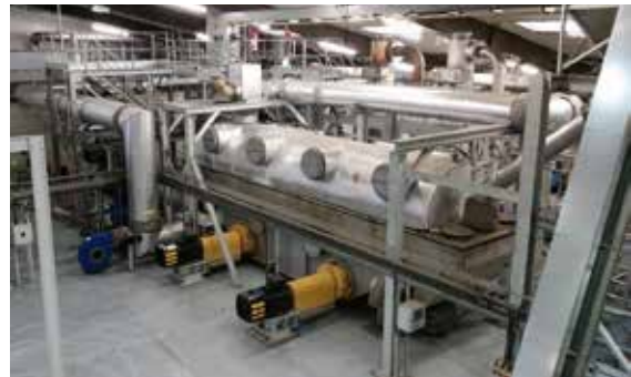
Torrefaction-reactor in R&D facility in Derby, England.
